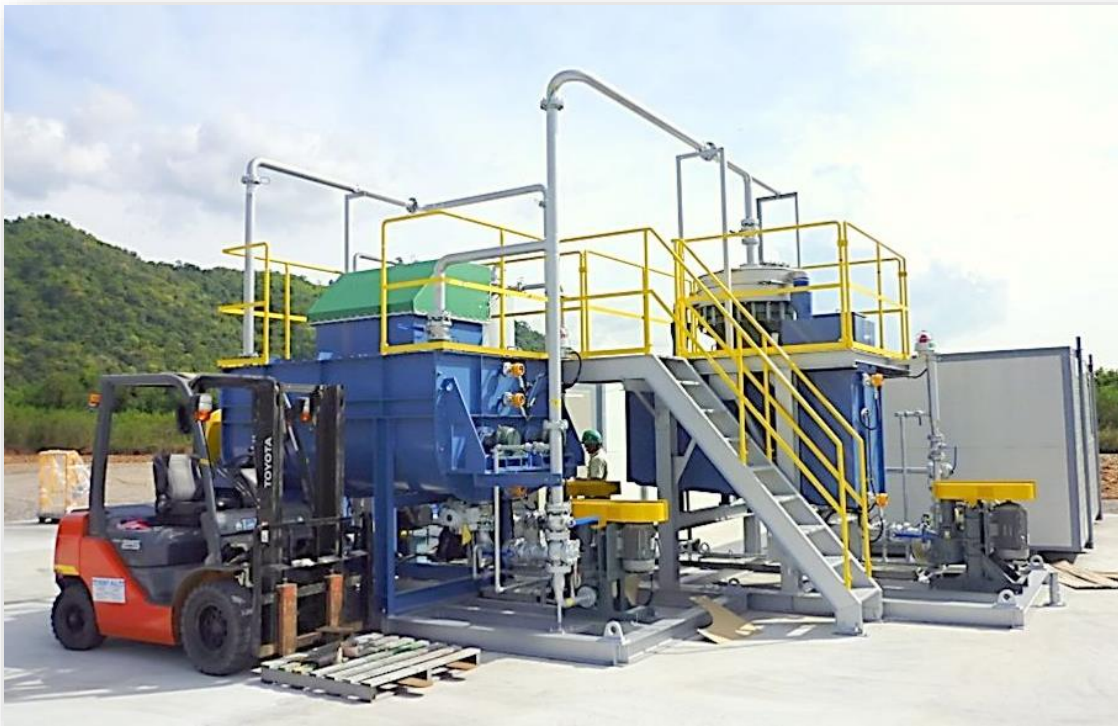
RF Pilot Plant
